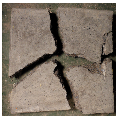
Fig. 11 Perpendicular crack pattern.
