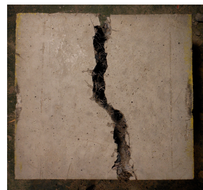
Fig. 12 Single-line crack pattern.
