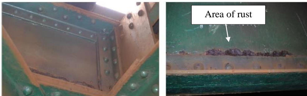
Fig. 1: The most common type of damage on steel bridges. (Rust on wall).
