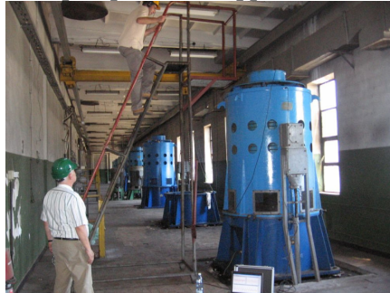
Fig. 1. Picture of the pump electrical motor
