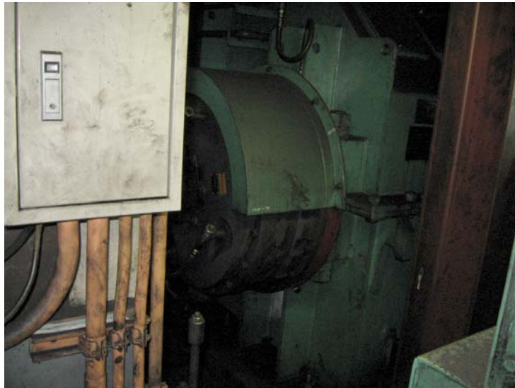
Fig. 3: Existing mechanical drive of the forging press.
