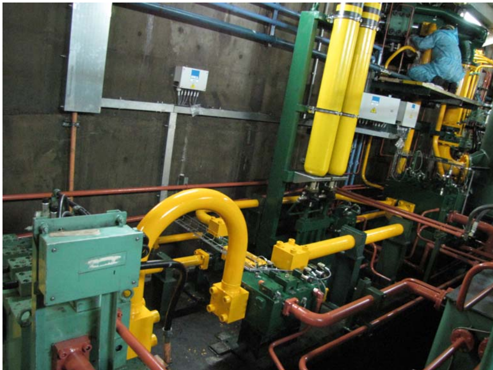
Fig. 5: New control manifold of new pump unit.
