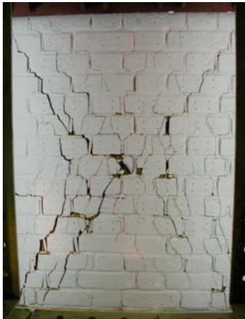
Fig. 7: Crack pattern at failure of the plain masonry control wall under a combination of vertical compression and cyclic shear.
