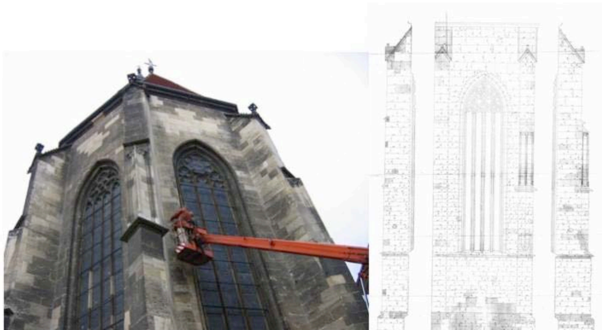
Fig. 1: Left - mapping and identification of individual building blocks, right - an example of existing paper facade plan (Vician et al., 1957).
