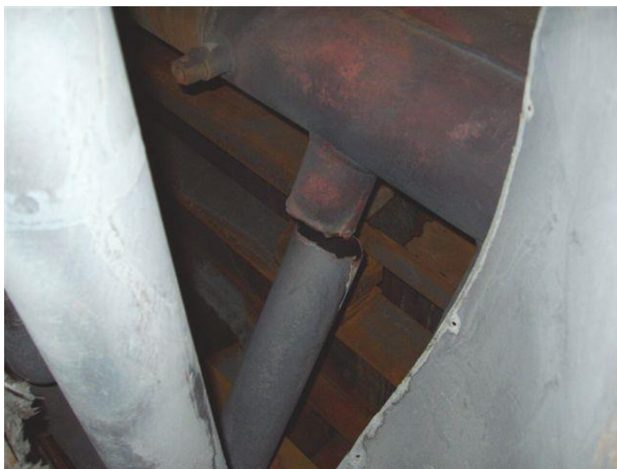
Fig. 1: Detachment of DN 100 connection piping in the area of welding to the chamber nozzle.
