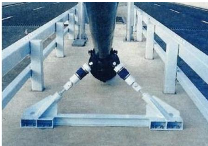
Fig. 8: Oil damper installed on the Aratsu bridge.
