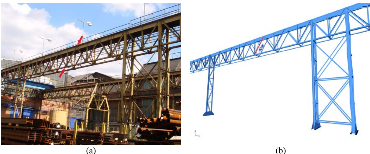
Fig. 1: Part of the supporting steel structure of the crane track. A realistic view (a) and model of construction with the marked diagonal B355 (b).
