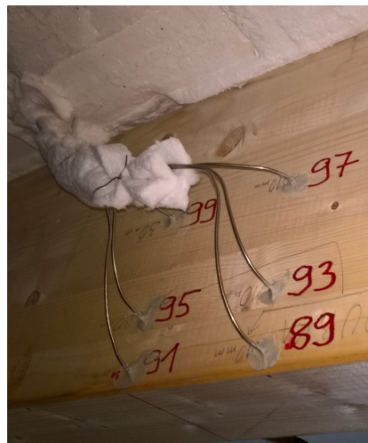
Fig. 4: Wiring to the sensors.
