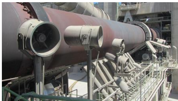
Fig. 1: Sintering zone in the rotary kiln with an open gear.
