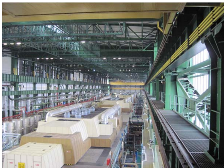
Fig. 1: View to the machine tool structures of the NPP with reactor VVER440/213.
